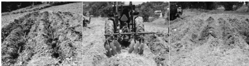
FIGURE 1. Field operations for installing tile drain and constructing ridges. Left: installation of tile drain at bottom of tilled plow layer. Center: construction of ridges over tile drain. Right: completed ridges.
