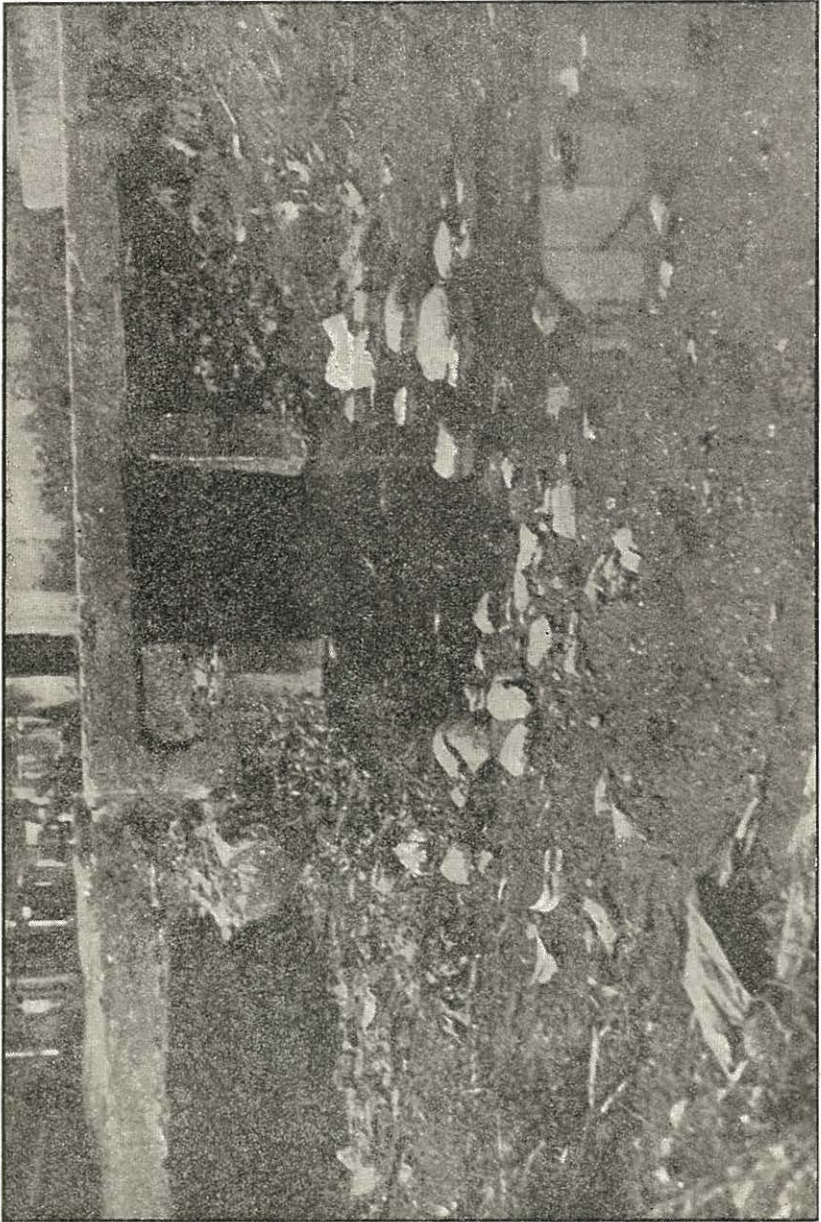
FIG. I.—Street culvert at Fajardo found to contain larvae of Culex quinquefasciatus .
